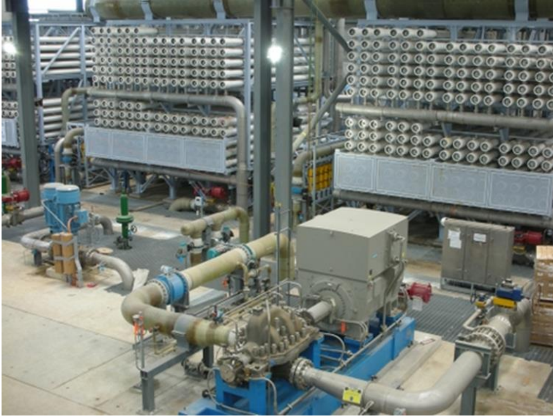
Fig 3.2: RO unit in Perth, Australia desalination plant (Sanz and Stover, 2007).
