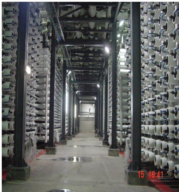
Fig 2.2: Ashkelon SWRO plant (Goichon, 2007)
